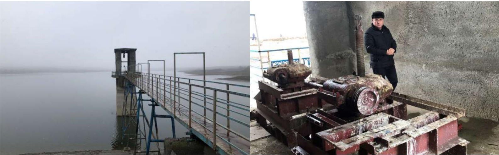
The valves of the intake tower of the Khachinchay dam are damaged and the dam's operator injured by an antipersonnel mine.
